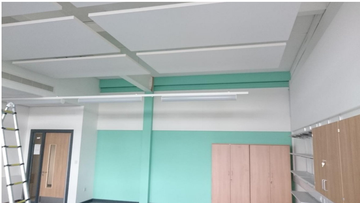
Figure 4: Small primary classroom with bulkhead for ventilation unit, rafts and wall panels
