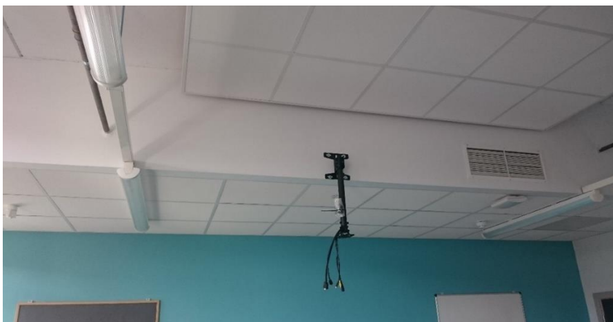
Figure 3: Bulkhead formed with MDF on upstand and ceiling tiles on room soffit
